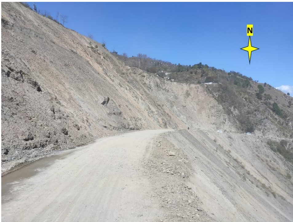
Figure 11: A view of Lohargali Landslide from Muzaffarabad-Garhi Habibullah Road.
